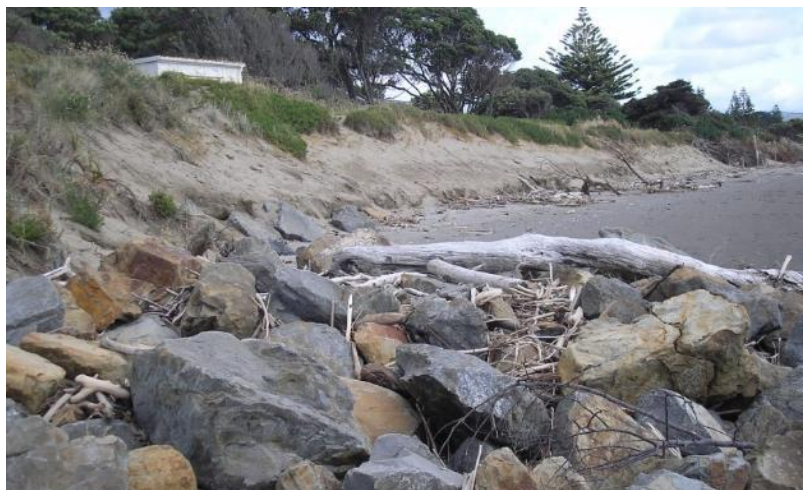
Southern portion of the Marine Parade rock toe revetment and adjacent shoreline.
